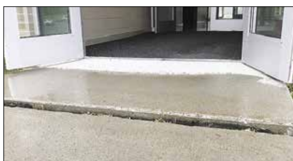
Uneven sidewalks at North Woods School are just one of numerous building construction issues in ISD 2142. photo by M. Helmberger
