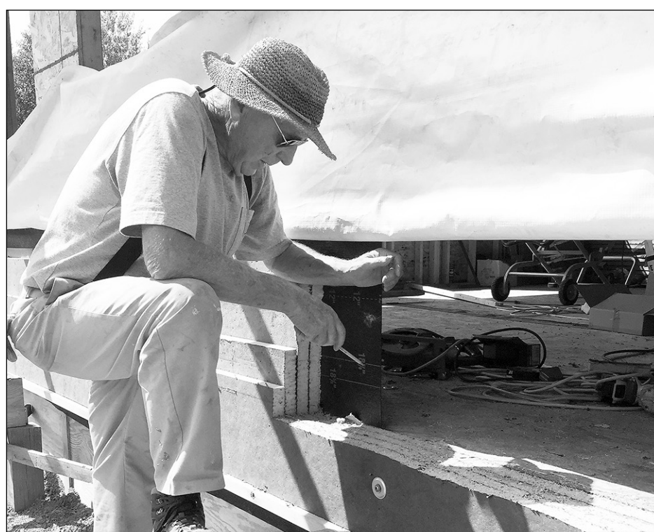
Andy Hill points to the vapor barrier, located behind the salvaged insulation sheets on the Perfect Wall. submitted photo
