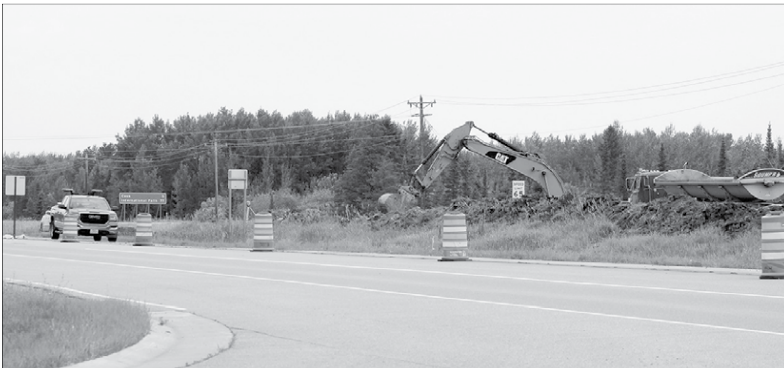
Construction crews excavate the median on Hwy. 53 at the intersection of State Hwy. 1 East and County Rd. 22 south of Cook Thursday afternoon. photo by C. DeY
