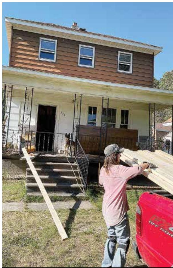
Left: The house, located on N Third Street, will see better days ahead.
