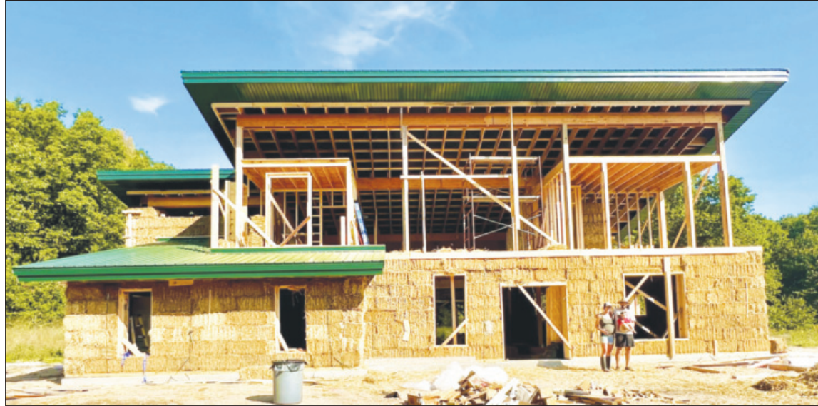
Mara Kalat-Brown and husband, Benjamin “Ben” Brown, stand with their son, Jupiter, in front of their home in progress that is being sustainably constructed with straw bales.
