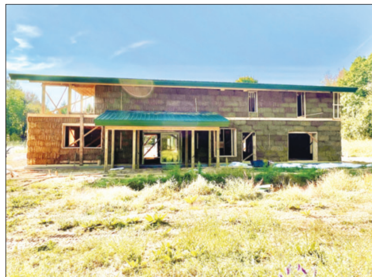
View of construction progress of Mara Kalat-Brown and Benjamin “Ben” Brown’s straw bale home being constructed in Harrison.
