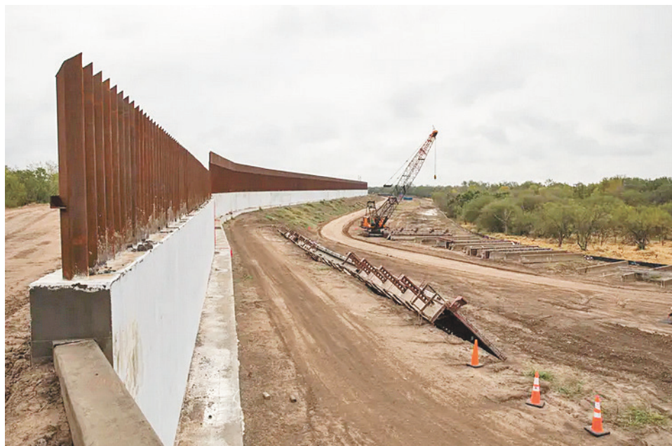
Construction on what the federal government says is a levee improvement project near Bentsen-Rio Grande Valley State Park in Mission on Jan. 12, 2022. Local immigrant advocates and environmentalists say the project is actually a border wall.
