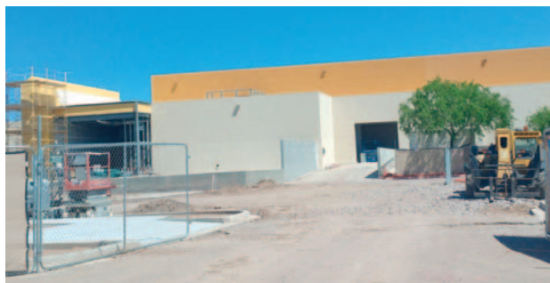
Work is expected to continue into August on the expansion of the Las Cruces Convention Center, 680 E. University Ave.
