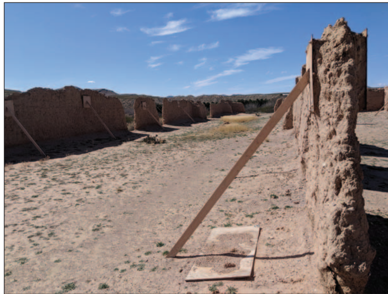
Preservation efforts are ongoing at Fort Selden. Posts help shore up crumbling adobe walls.
