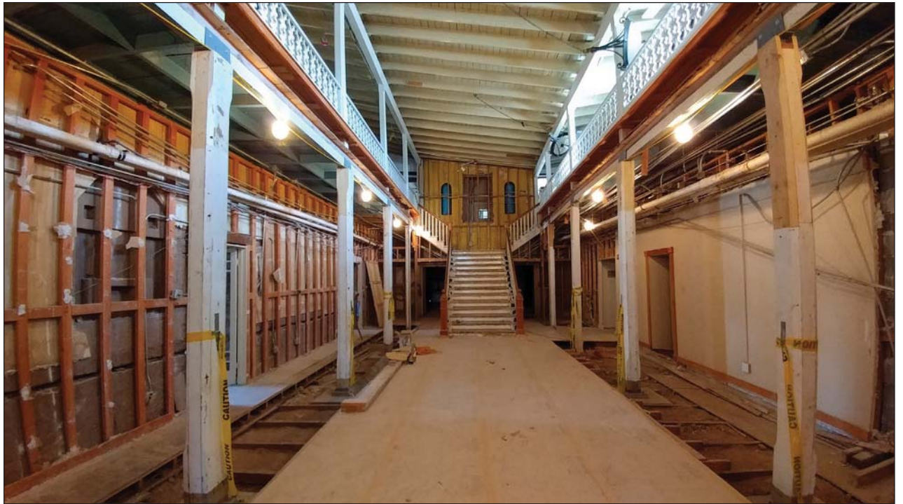
An interior shot of the historic Amador Hotel as renovation continues on the city's oldest property. The hotel was built in the 1870s by Martin Amador, patriarch of one of Las Cruces' oldest and most influential families.
