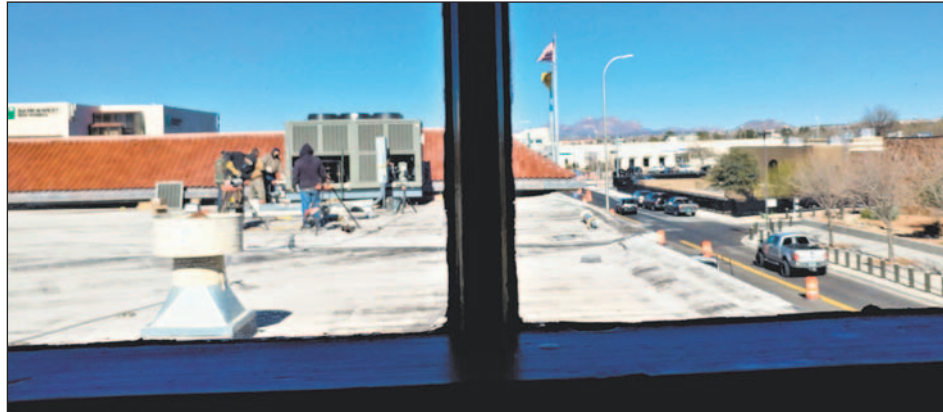
A new HVAC system is being installed on the roof of the old courthouse building.
