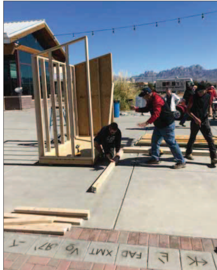
DACC Building Construction Technology students build a structure at the Las Cruces Home Builders Association Home and Garden Show Feb. 24-25.
