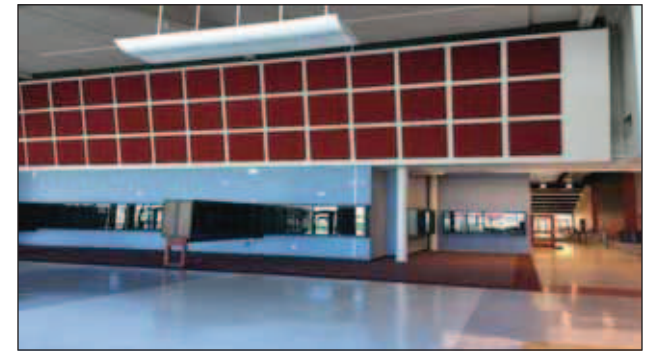
Interior work is ongoing in the lobby of Las Cruces High School's main gymnasium.
