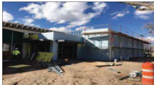
An expansion and remodeling of the school kitchen is underway at Mayfield High School.
