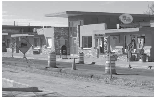
The Emporium remains open during its regular hours as construction continues on Water Street outside the store as part of the downtown Church-Water conversion project.
