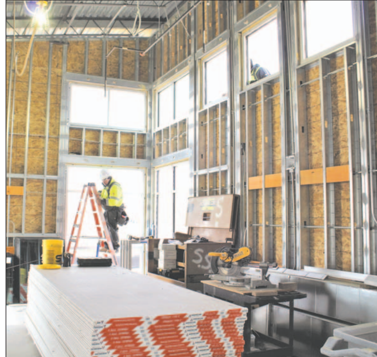
Construction of the City's new LEED-Certified Water Quality Laboratory at the JHWTF at 2851 W. Amador Avenue is on schedule.
