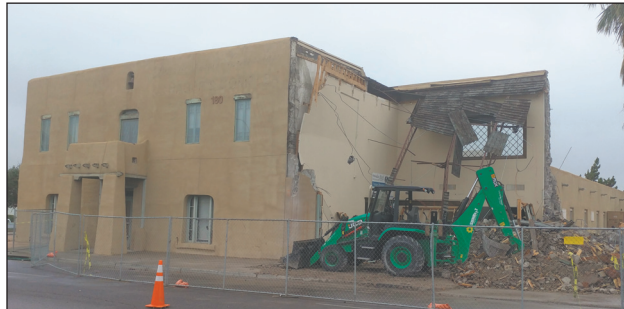
Phase three of the Amador Project, currently underway, is the demolition of the non-historic parts of the Amador Hotel.
