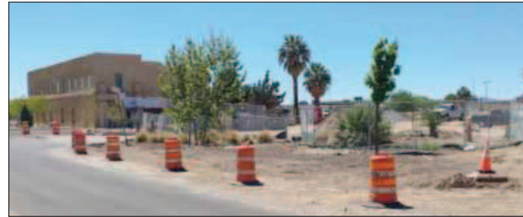
The former site of My Brother's Place is now fully under construction as part of the Amador Hotel renovation project.
