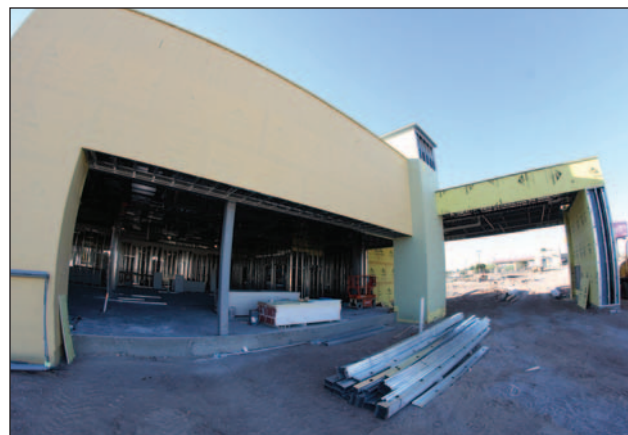
MountainView's new ER facility is being built at a cost of more than $10 million.
