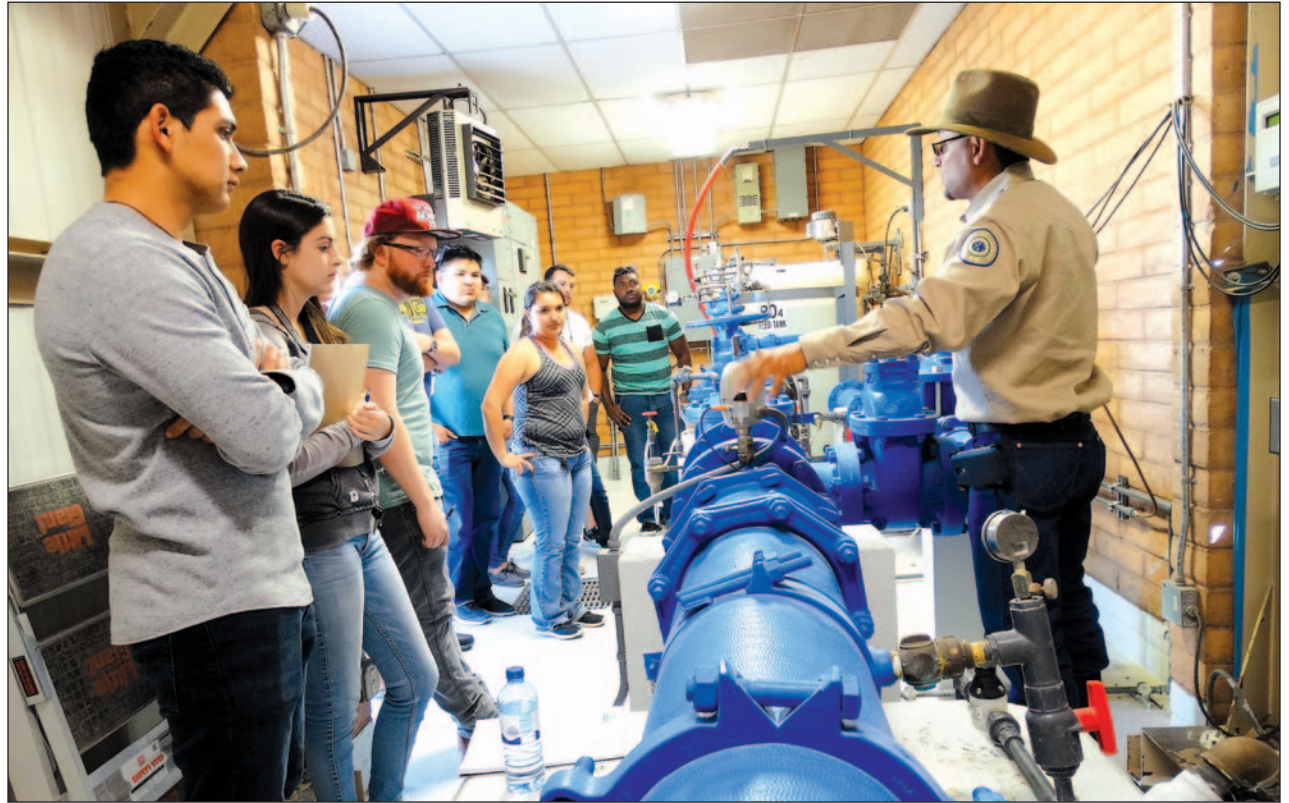
Pascual Rodriguez, water production supervisor, introduces NMSU engineering students to the inside of an LCU water well building.
