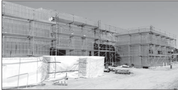
Renovation of Las Cruces High School, the city's oldest high school, is expected to be completed in 2018.
