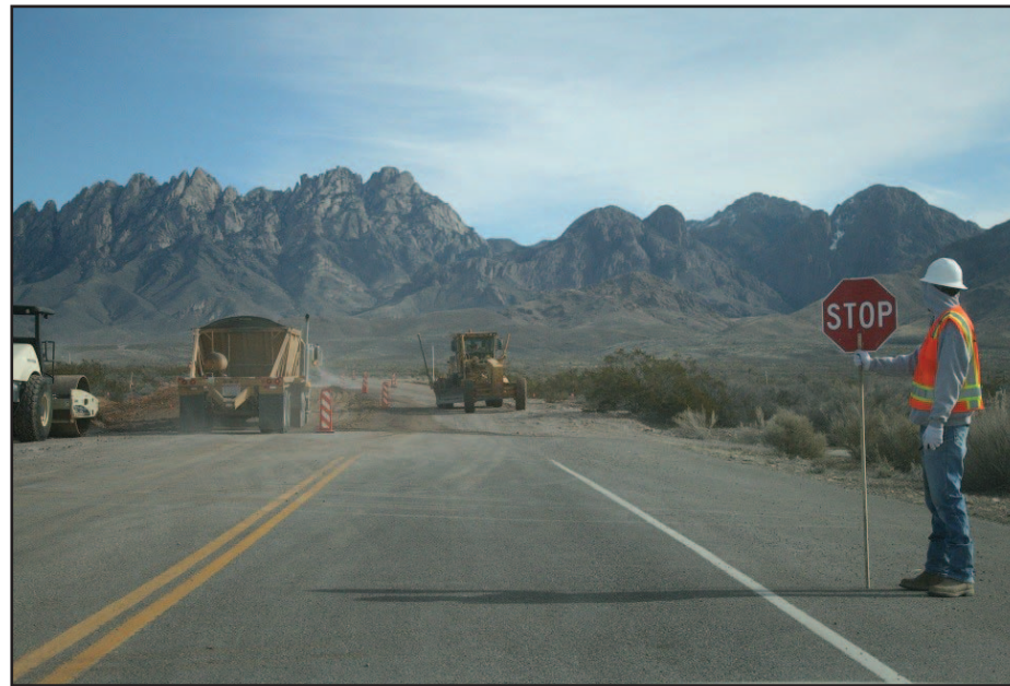
Jesus Rincon of Mountain States Construction stops traffic on Dripping Springs Road while drivers wait for the pilot truck to return and allow them to continue their eastbound journeys.
