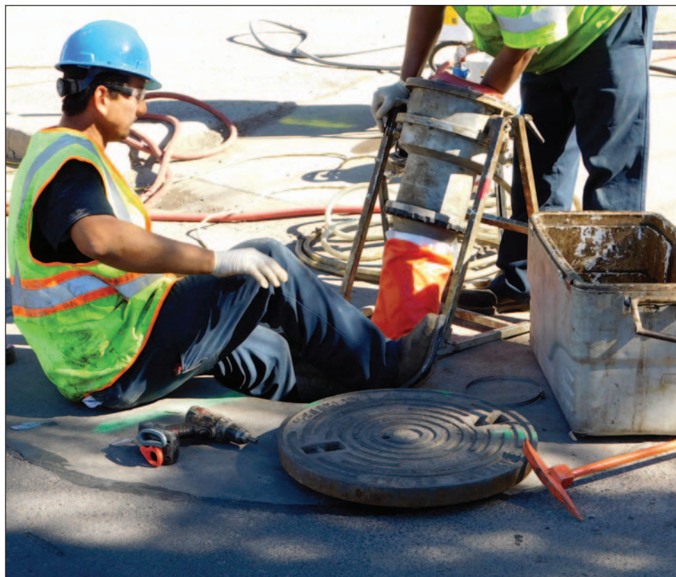
The cured-in-place sleeve, or pipe within in a pipe, is inflated to tightly fit the aging sewer pipe, leaving it better than new.
