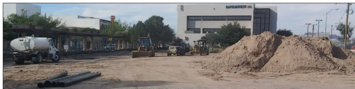
Work began in the summer of 2015 on the long-sought city plaza in Downtown Las Cruces.
