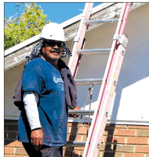
Jesus Rodriguez of CRS, a Las Cruces commercial roofing company, works on the roof of Mesilla Valley Center for Dental Medicine at 608 S. Alameda Blvd. Roofers were in high demand during the first half of 2016 as building owners looked to repair damage from October 2015 hail storms.
