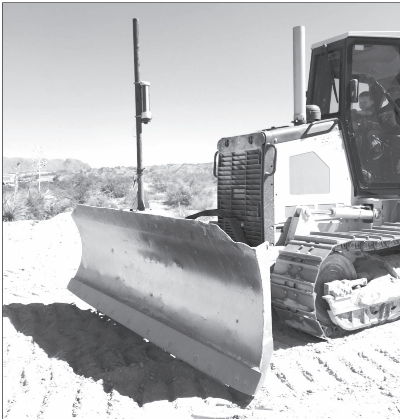
Gallardo Construction broke ground with a bulldozer in the desert on March 14. A pole in the background holds a receiver which works in conjunction with a spinning laser beam (attached to a pickup truck) that informs the bulldozer of the necessary grade.
