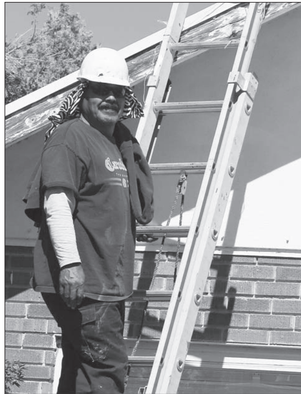
Jesus Rodriguez of CRS, a Las Cruces commercial roofing company, works on the roof of Mesilla Valley Center for Dental Medicine at 608 S. Alameda Blvd.
