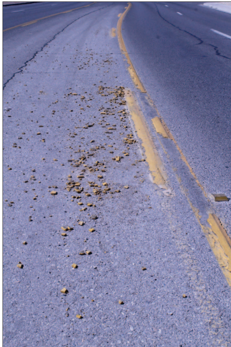
Some yellow lines on the roadways in Las Cruces are cracking and leaving piles of paint chips.
