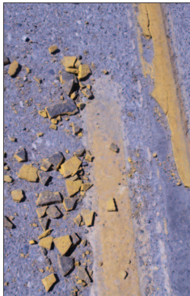
The cracking yellow lines on some of Las Cruces’ streets are caused by a combination of dry air, lack of rain and impenetrable surfaces.
