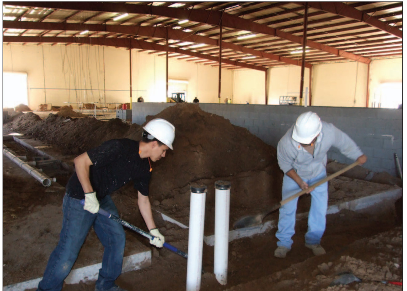
Interior renovations have begun to transform the vacant building at 875 W. Amador Ave. into a tortilla factory for Franco Whole Foods of California. Pictured are Gabriel Nerios and Juan Morales of C.D. Mechanical of Las Cruces installing a portion of the extensive drainage system the factory will require.
