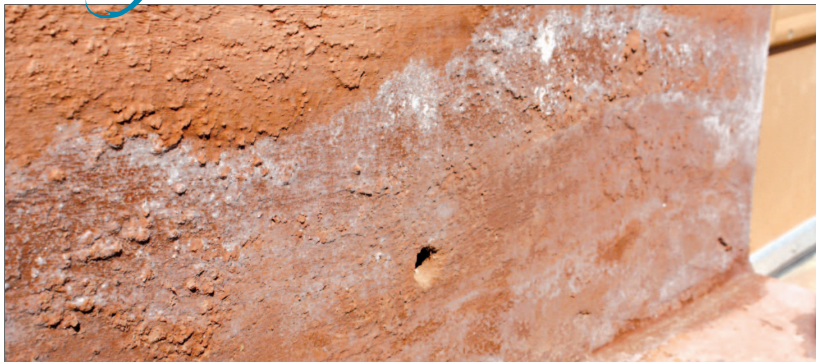
Efflorescence, a process that may indicate damaging levels of salt in porous building materials such as adobe, stone and other types of masonry, appears as a salt rime on the surface of a wall as salt crystals migrate out of the material.
