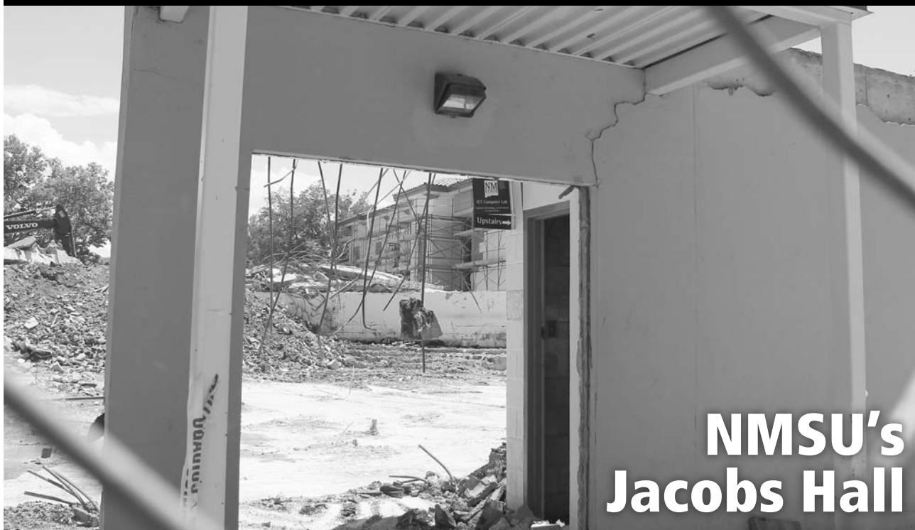
Jacobs Hall on the New Mexico State University campus has been torn down to make room for new structures. Located between Hardman Hall and the former Hershel Zohn Theatre, Jacobs Hall housed the university computer labs, but was built in 1963 as a fine arts and music building.
