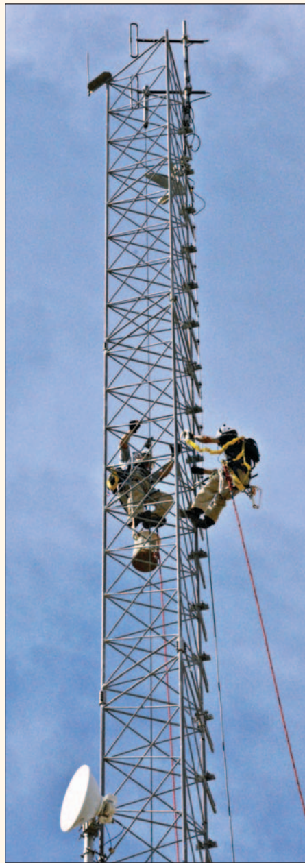
Doña Ana County radio technicians William Tamplen, right, and Brad Sacca work to install a folded dipole antenna that will collect and transmit information from several flood
