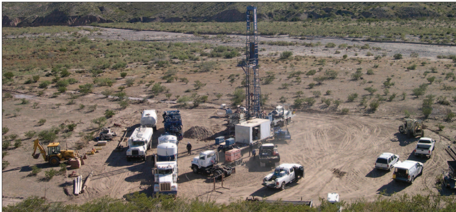
The Hatch village test well site was photographed Nov. 5 by geologist Jim Witcher while a crew from Baker Hughes of Farmington cemented a surface casing, a process required by the New Mexico Office of the State Engineer if there is any potential for artesian water or water under pressure to leak.
