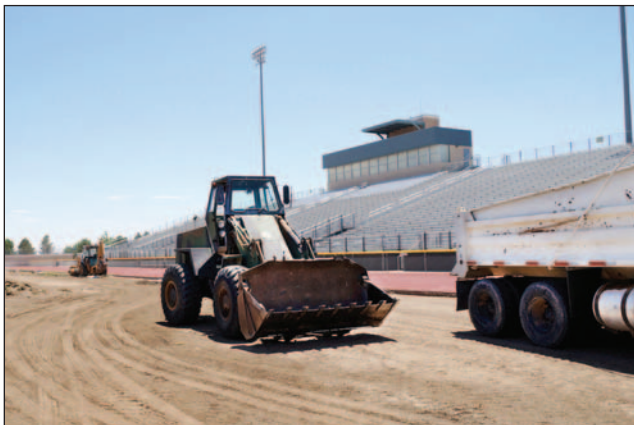
Work to replace the grass at the Field of Dreams with artificial turf was under way in July.
