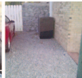
Completed 5 Ton System
