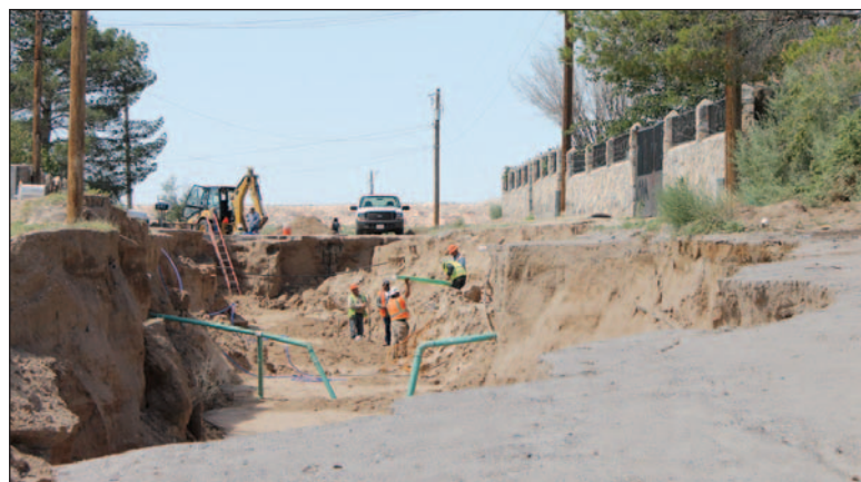
County work crews begin sorting out underground pipes on a street in La Union that was demolished by flood water after an earthen dam gave way due to heavy rains last week.
