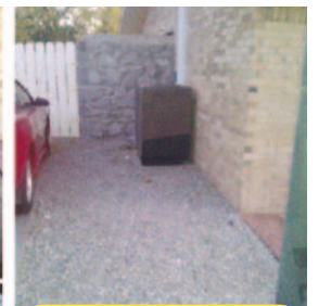
Completed 5 Ton System
