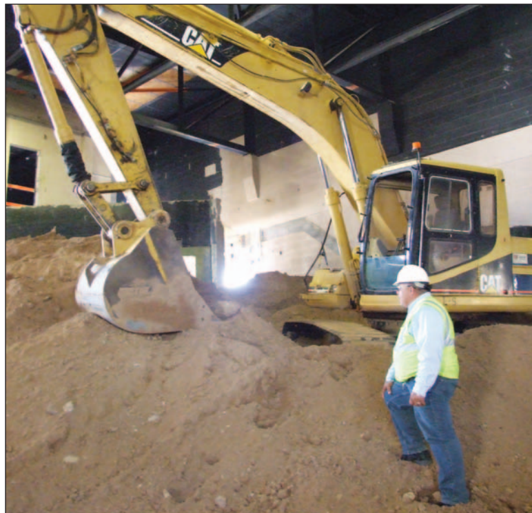
Inside the former Hershel Zohn Theatre, an advanced technology classroom is being constructed for NMSU as part of Peter V. Domenici Hall, a complex of new and renovated space that will house the former senator's papers, as well as classrooms and offices. Construction got underway in July and is scheduled to be completed in July 2014.
