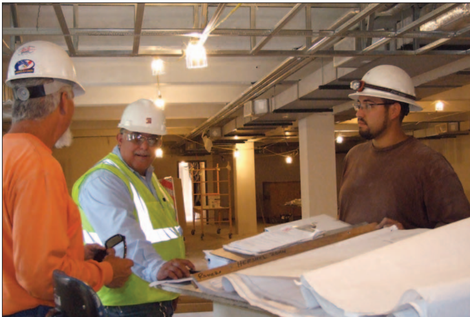
Foreman Paul Coleman of Carver Electric, project manager Jon Padilla of New Mexico State University and apprentice Albert Hernandez review plans in the Branson Library area, where renovations are nearing completion.
