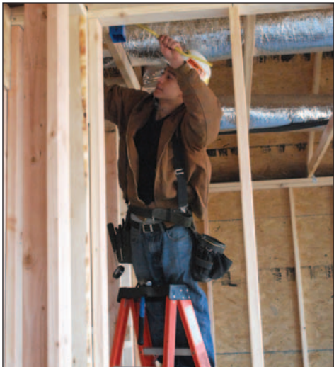
Aaron Sanchez, a third-year apprentice, handles wire that will be used for a smoke detector.
