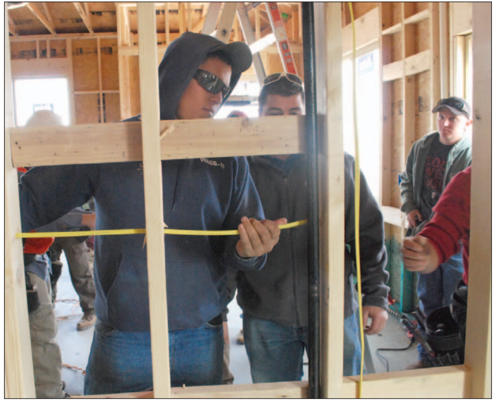
Third-year apprentice Brooks Roberts helps wire the kitchen circuits as journeyman Richard Gray watches. Apprentices spent about two days doing the rough-in electrical work on the home.
