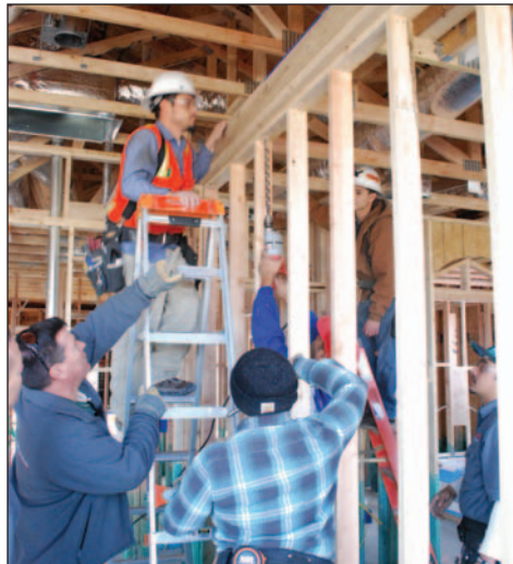
Mike Gray shows a group of apprentices where they need to drill so the living room circuit can be completed.
