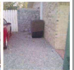
Completed 5 Ton System
