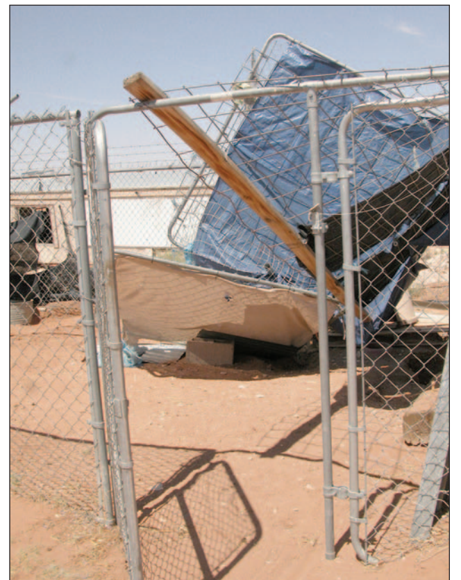
Las Cruces Bulletin photos by Todd Dickson The “roof” of this animal holding pen where Doña Ana County keeps animals in criminal cases collapsed during a storm late last month. Located in a secluded area outside Las Cruces city limits, the cages are all in the open, with limited shelter from the elements.
