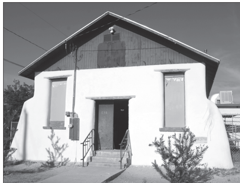
Great strides have been made in the Phillips Chapel restoration project. Volunteers hope to have the structure completed by the end of the year.
