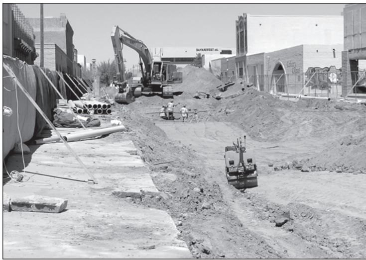
March 27: Crews install a sanitary sewer line at the intersection of Main Street and an alley.
