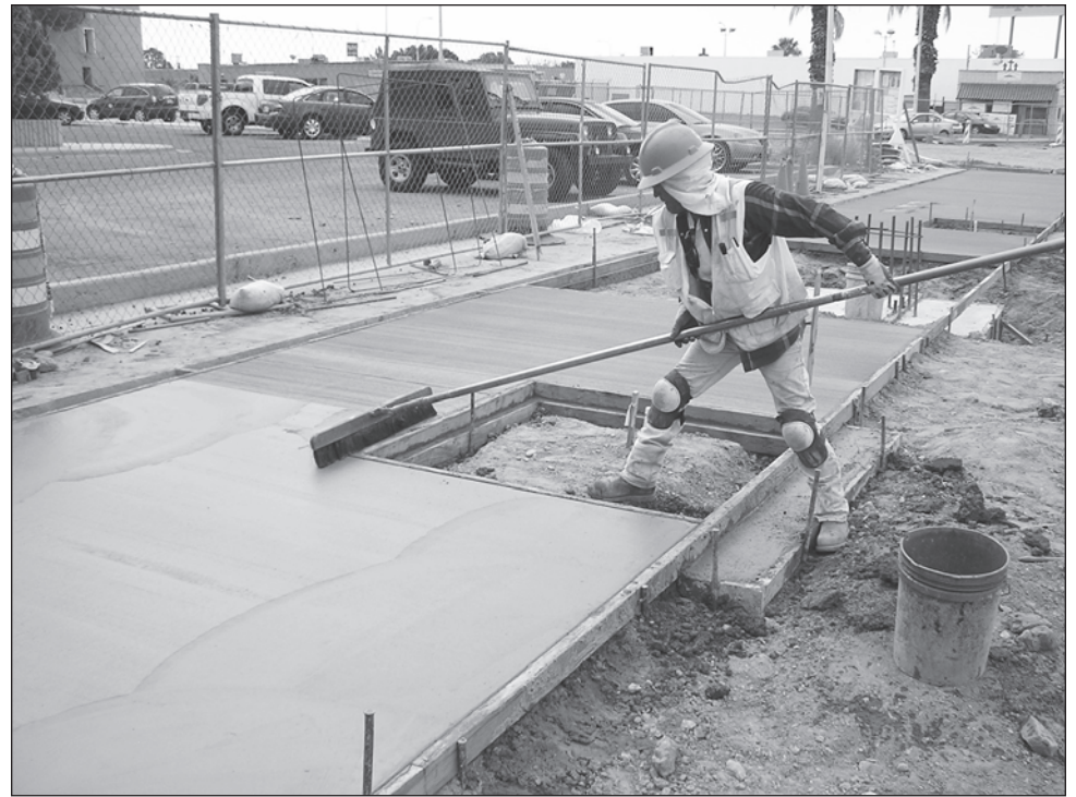
Aug. 8: Anacleto Cervantes broom-finishes the colored concrete sidewalk near the south end of the project.
