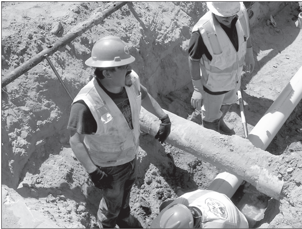
March 26: Jose Luis Solis, Roberto R. Avalos and Jose Orozco Gonzales install the sanitary sewer main line for the final phase of Downtown Main Street reconstruction.
