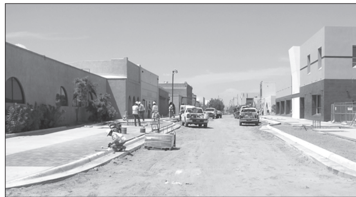
Construction continues at the New America School at right and on Main Street.
