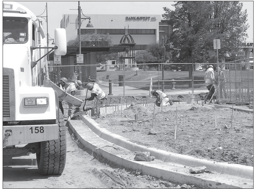
Curb work in progress near Bank of the West during recently completed Main Street reconstruction.
