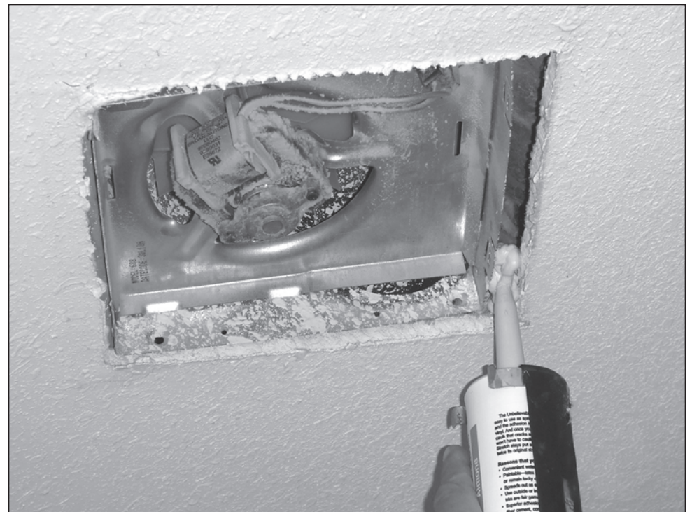
Extra caulking around the opening of your vent fan will help it work more efficiently.
