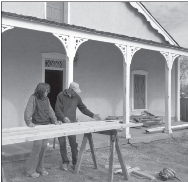
Sonya Cooper and Gregg Henry cut timber for structural shoring at the Nestor Armijo House, which is being renovated by the Las Cruces Chamber of Commerce with the help of MVP. It will be part of the home tour.
