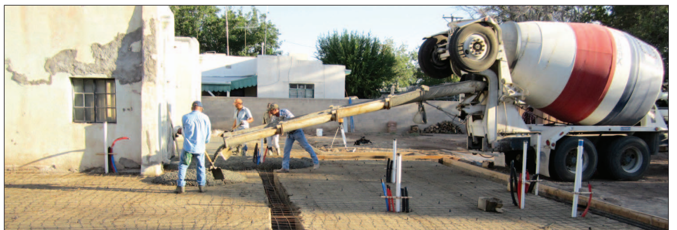
Workers lay the foundation for the addition of the home during the beginning stages of the renovation.
