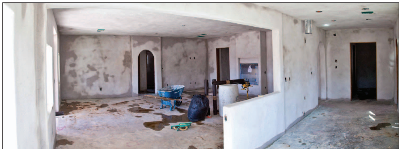
Still a work in progress, the great room and kitchen area are awaiting a final coat of traditional lime plaster.
