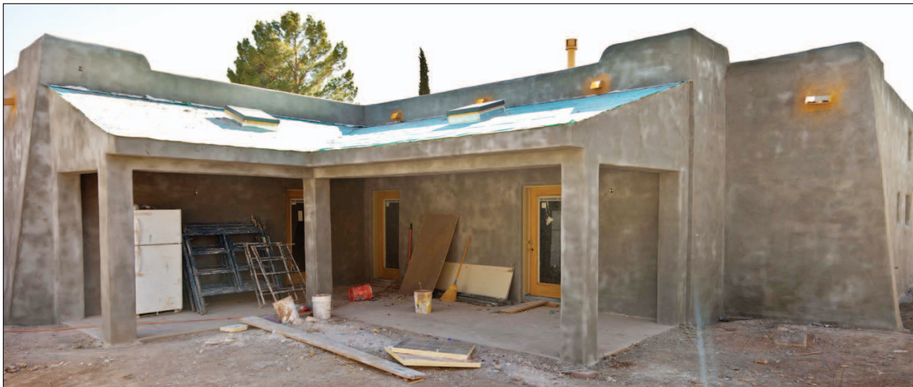
Built in 1949, the home at 730 N. Miranda St. is in the process of being renovated into a LEED-certified creation.
