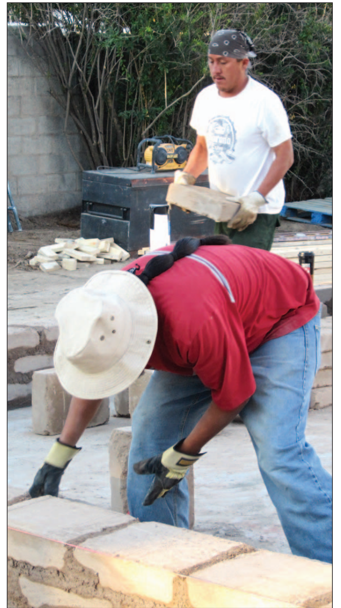
Craftsmen from the Santa Domingo Pueblo lay adobe bricks during the renovation of the home.
