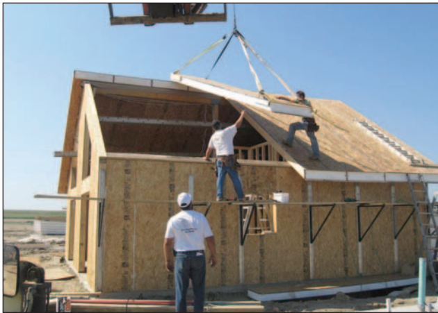
NetSolar Construction workers piece together the structural insulated panels of a home. The panels create a tight exterior envelope, making them green and energy efficient.
