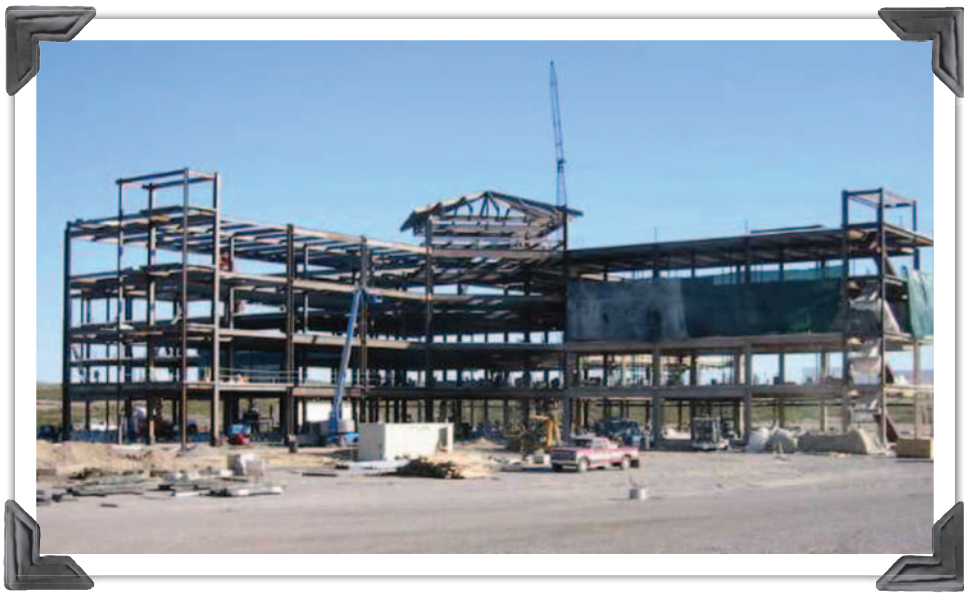
Construction begins on MountainView Regional Medical Center, after the announcement was made in July 2000 that Las Cruces would be getting a second hospital.
