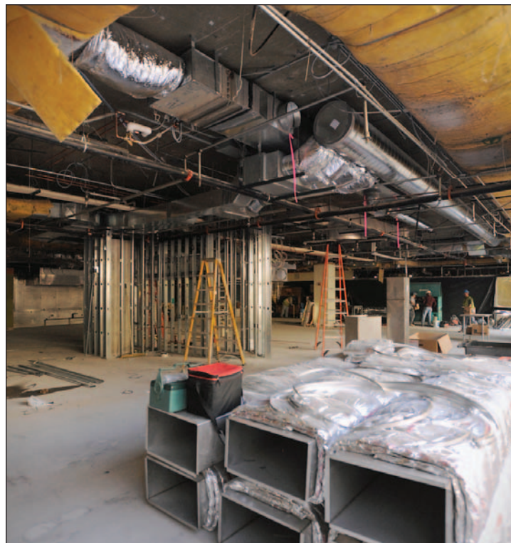
Workers made major renovations to the Taos Restaurant in the Corbett Center Student Union this summer at New Mexico State University. The $3.7 million in renovations included new stone work.
