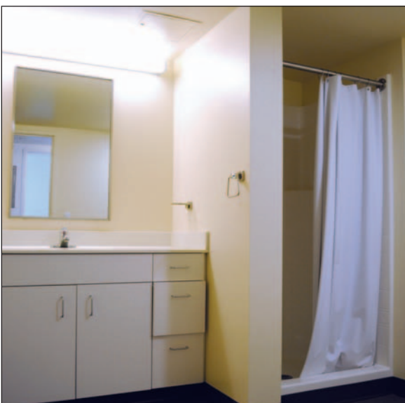
Motion sensors turn on the lights in the bathrooms.
