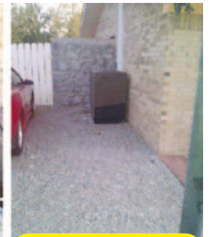
Completed 5 Ton System
