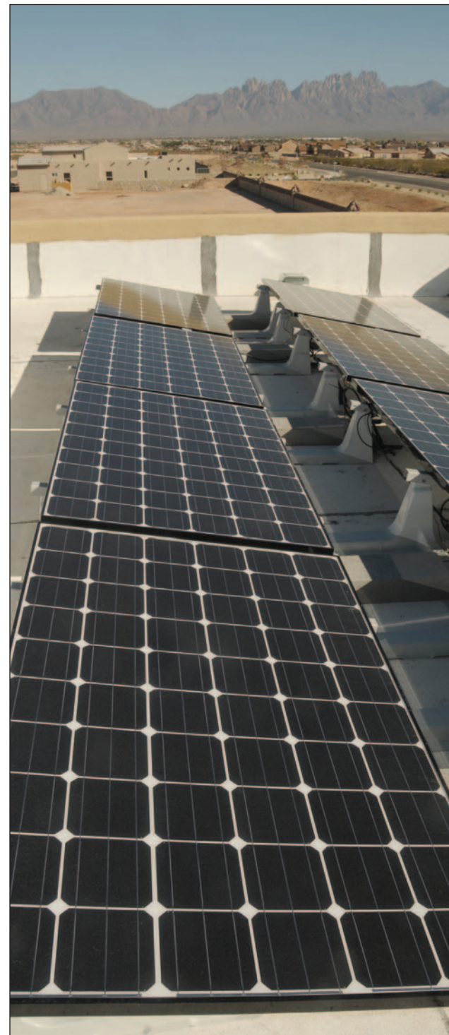
Solar panels line the roof of the 2,526-square-foot home.
