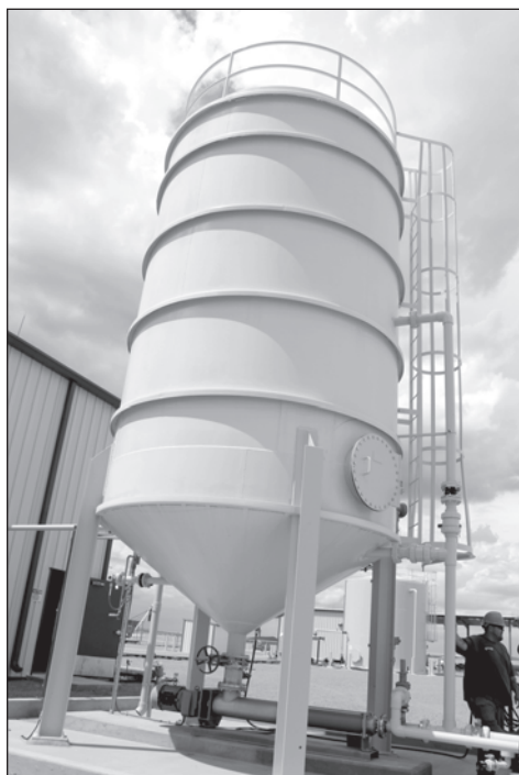
This tank at Sapphire's Columbus, N.M., facility holds 15,000 gallons of "green crude."
