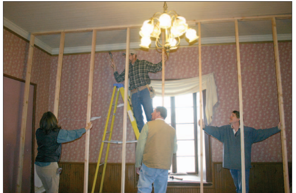
MVP board members Sonya Cooper, Gregg Henry and Eric Liefeld work with the Greater Las Cruces Chamber of Commerce President Richard Haas to erect structural shoring at the Nestor Armijo House.
