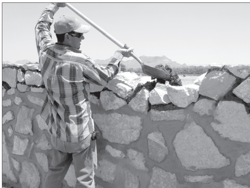
Ever Rivera, who has worked for the company for eight years, adds another piece to the puzzle of a rock wall for E&R Contractors.
