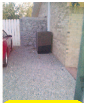
Completed 5 Ton System
