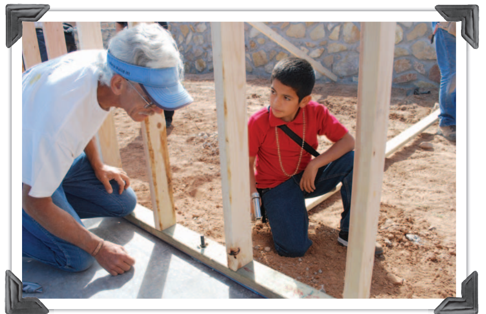
MVHFH Construction Supervisor Steve Blyth helps Joshua Covarrubia tighten bolts of his future home in 2010.
