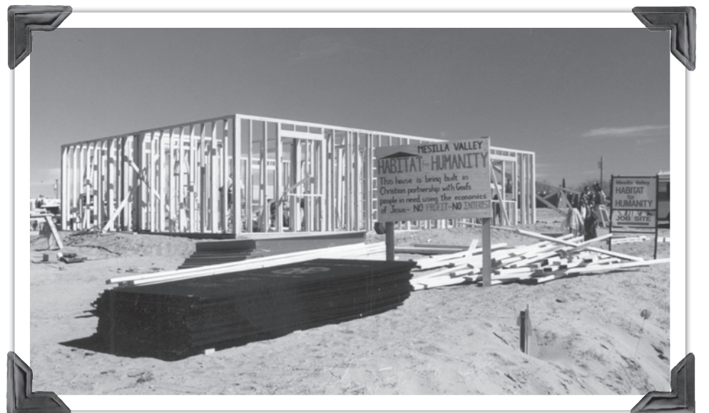
Home No. 5 built by the nonprofit organization begins to take shape. During the past 25 years, 88 homes have been built by MVHFH.
