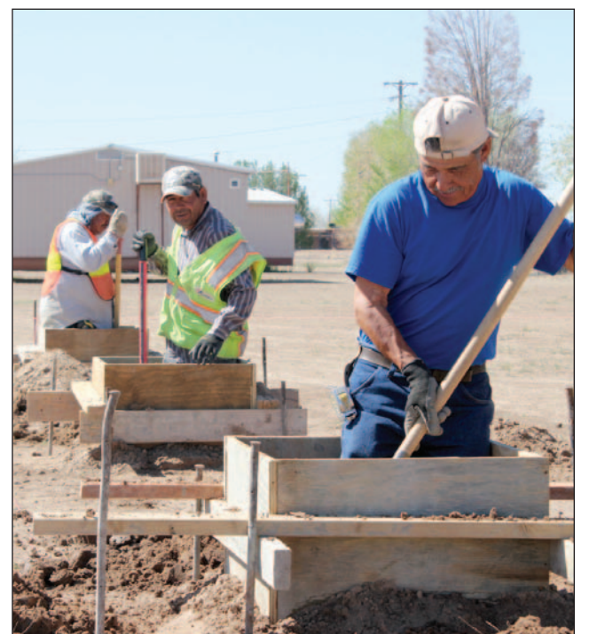
Geraldo Gomez, Erasmo Onchonda and Jose Mendoza of Morales Construction prepare the foundations for the new portable buildings at Las Cruces Catholic School.
