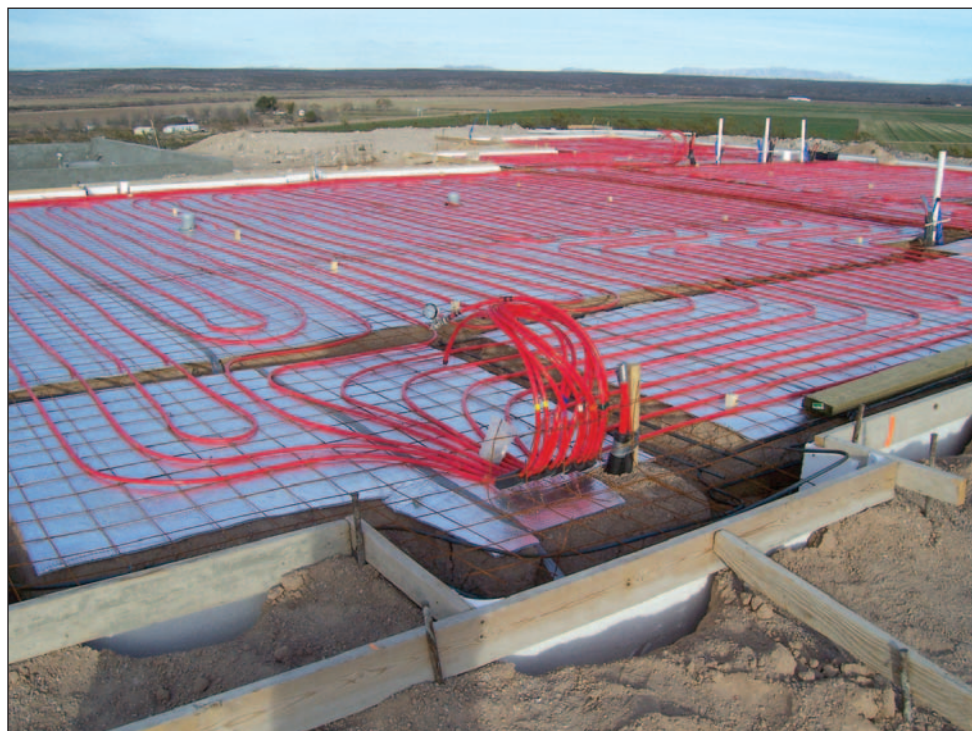
Radiant heating designed by Sun City Plumbing & Heating runs along the foundation of a home under construction.
